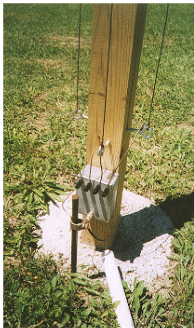
Figure 3—Near the base of the center pole, an aluminum enclosure houses the four relays. The four wires from the top of the pole are anchored at the pole base in large eye-bolts, one on each face of the pole. Each wire's bottom end connects to the inside of the relay box through binding posts. From the hidden pole face, the wire passes through a hole drilled in the pole near the eyebolt above the relay box. The feed line approaches the pole through a piece of PVC pipe and is attached to the box via a BNC connector. A ground rod connected to the relay box finishes the installation.
